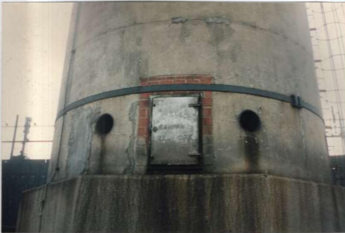
Photo #2 - View of access door at the base of the chimney. Concrete column is solid & sound.
