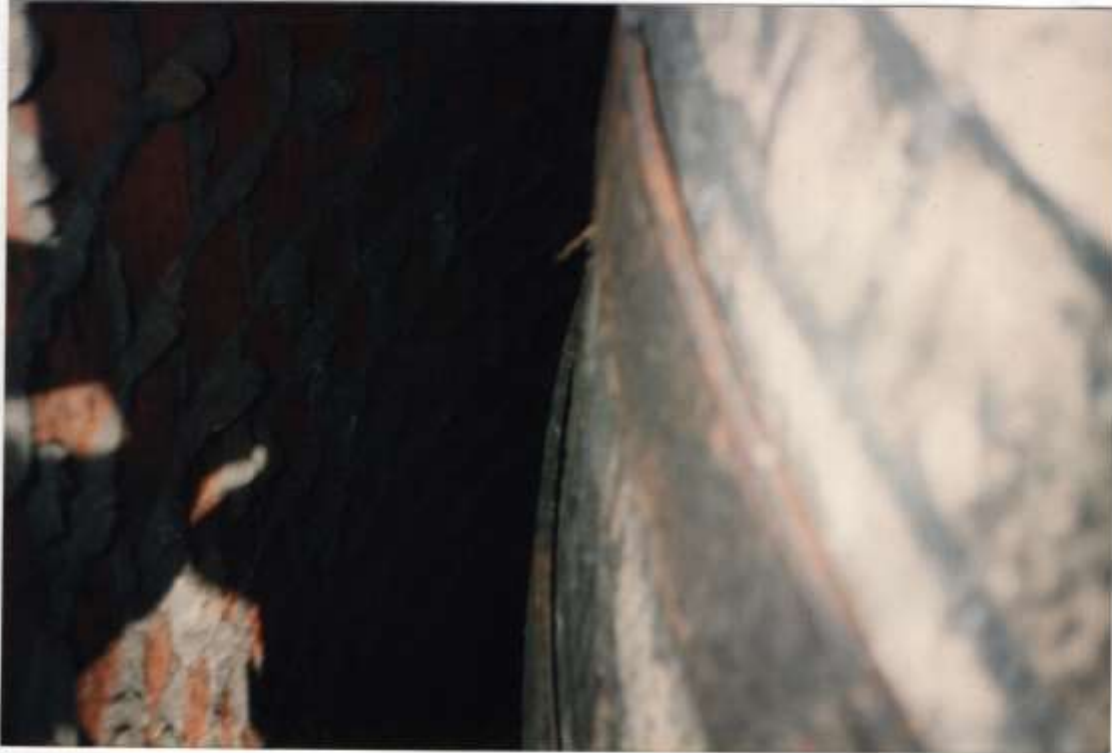
Photo #38 - View into the air space between the liner and column interior. Brickwork is solid & sound.
