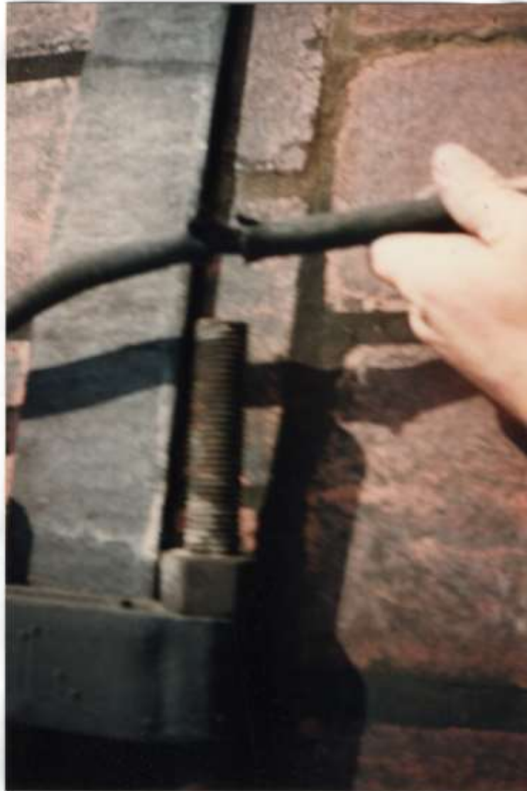
Photo #31 - The lead coating covering the Lightning Protection system cable was found cracked and split open in several areas throughout the top of the chimney.
