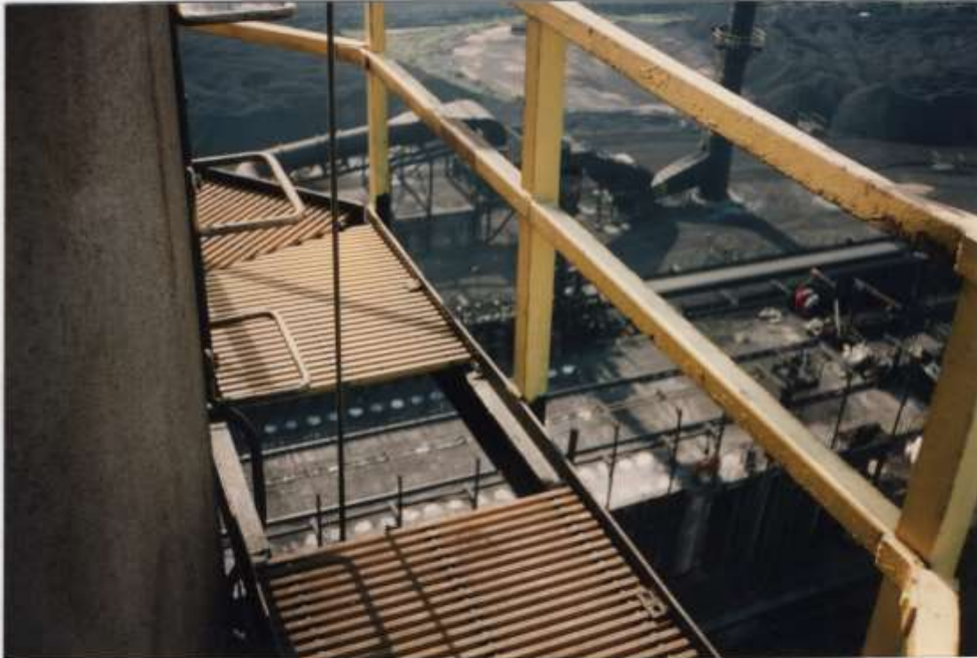
Photo #12 - South quadrant, typical condition of platform at midpoint of chimney. Minor rusting of hand rails noted.
