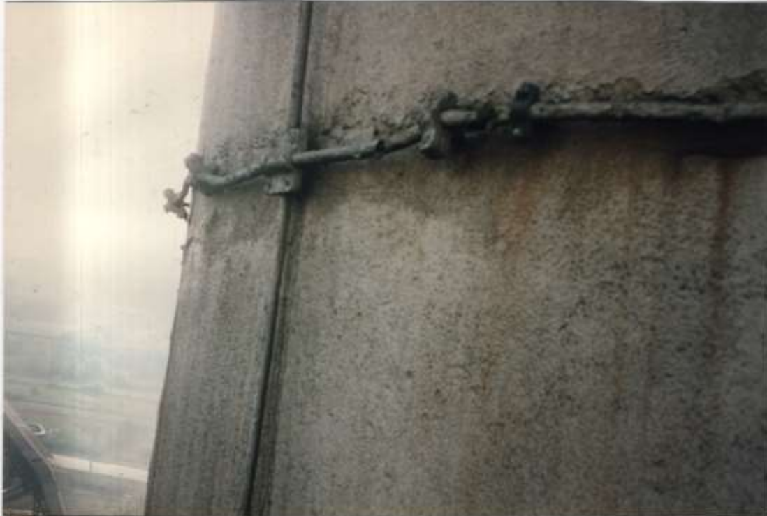
Photo #8 - Midpoint circular cable at connection to downlead, west quadrant. Note broken anchors.
