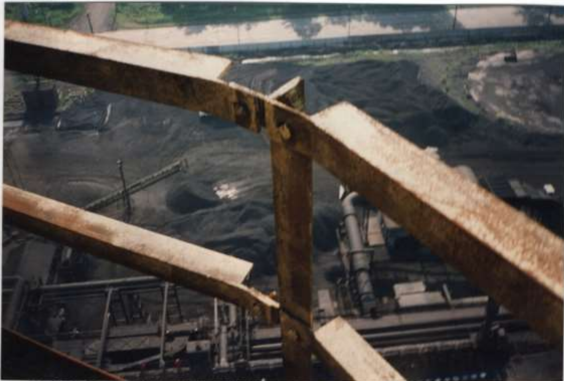
Photo #25 - Close up view of the top platform handrail. Note the steel is rusting freely.
