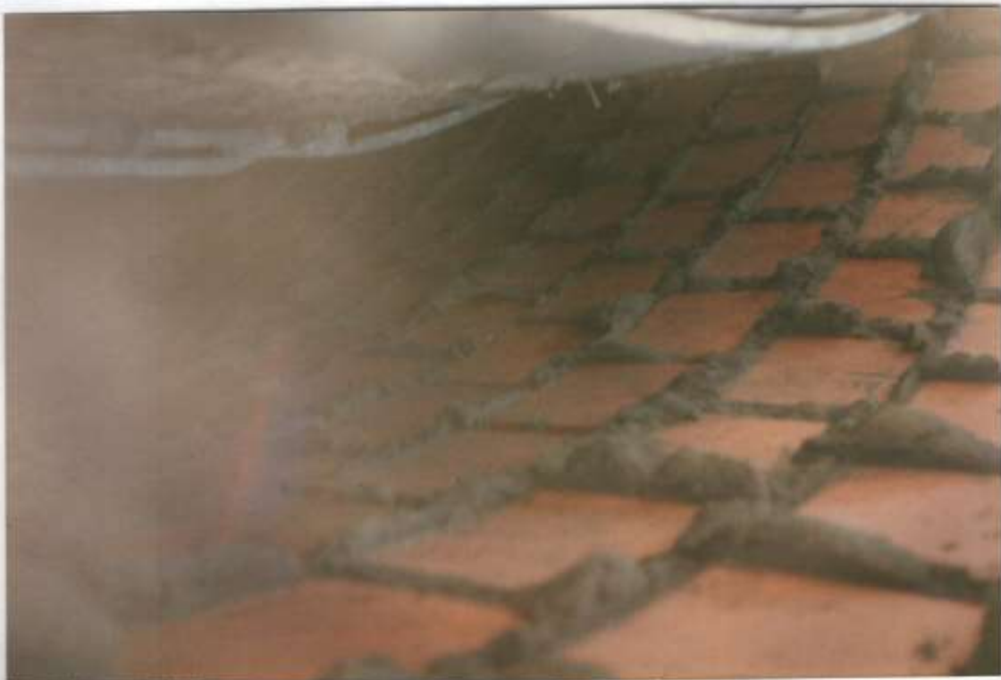
Photo #37 - View into the air space between the liner and the column interior. Brickwork is solid & sound.
