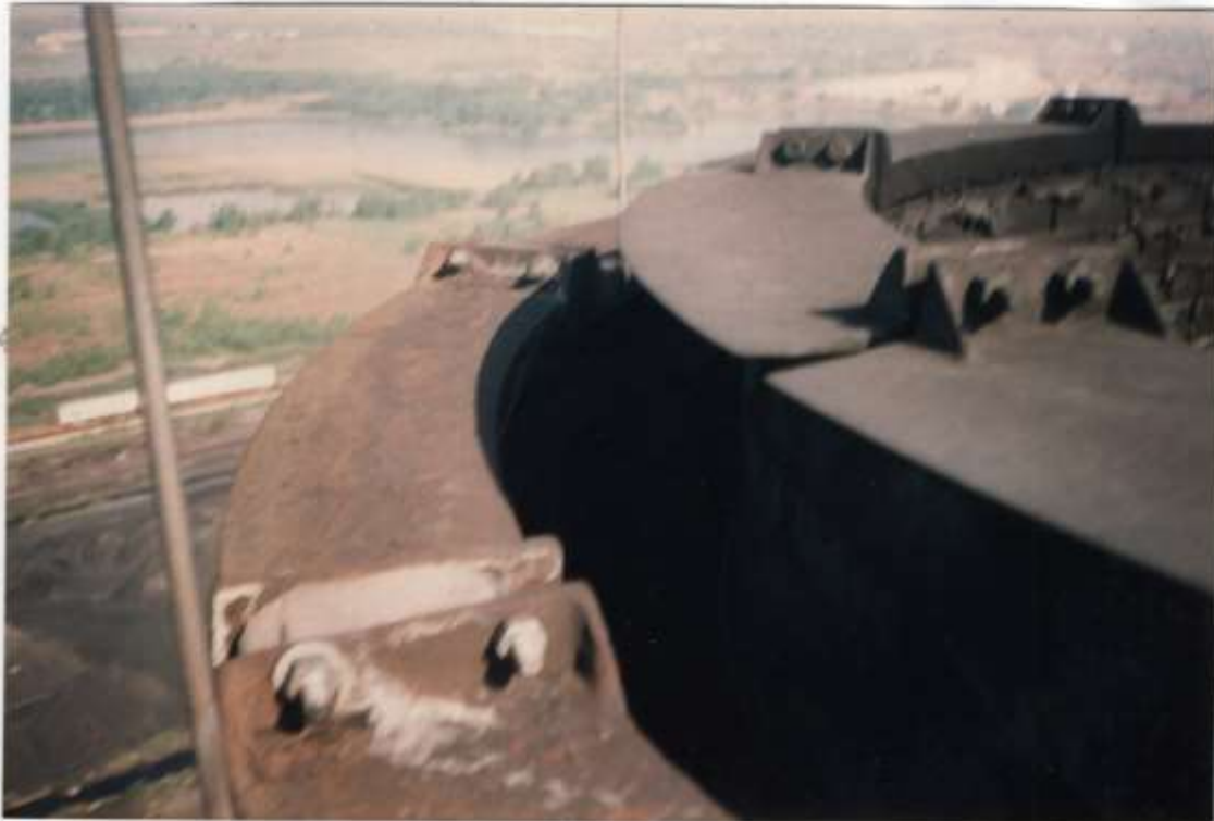
Photo #32 - Column & liner caps are intact. Note minor corrosion & rusting conditions.
