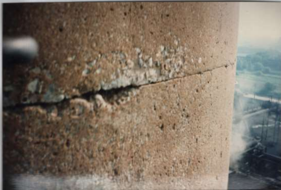
Photo #7 - Open construction joint at the 80' elevation, right of the step irons.
