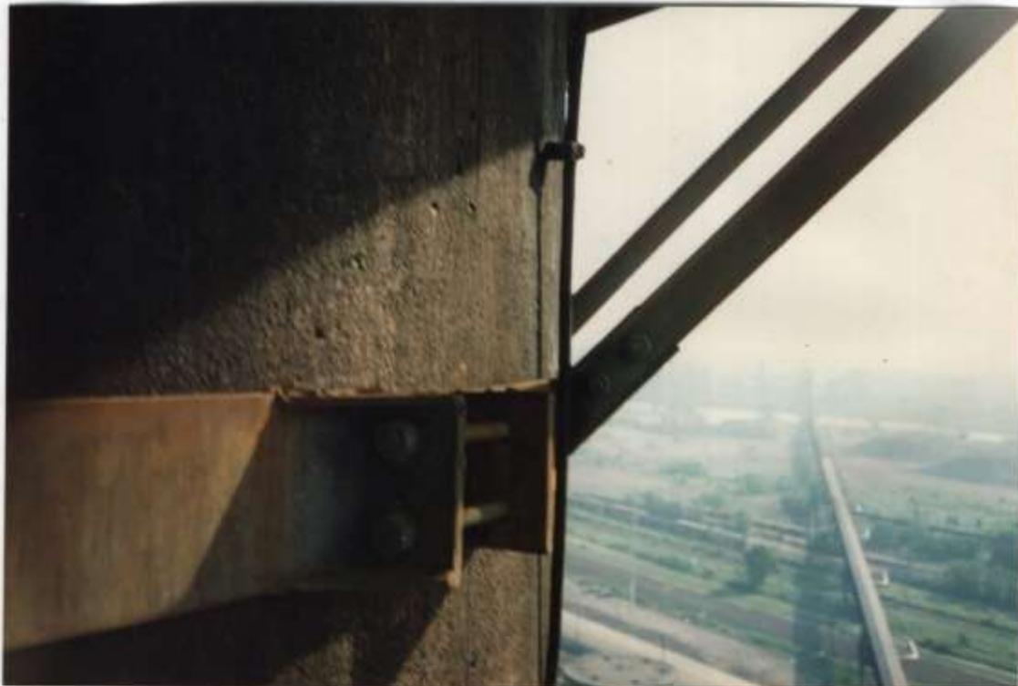
Photo # 18- The support band and bottom support angles for the top platform are all solid & sound. Minor rusting noted.
