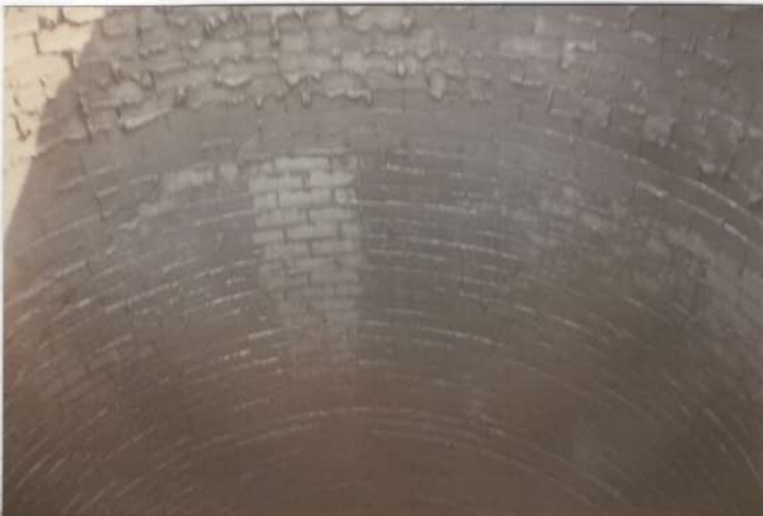
Photo #39 - View looking into the top of the liner. All brickwork is solid & sound.
