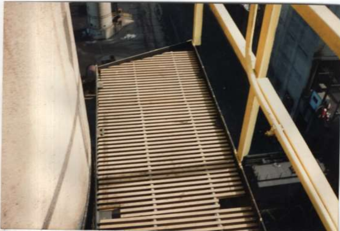
Photo #11 - Typical condition of platform at midpoint of chimney on the east quadrant. Platform is safe & sound.
