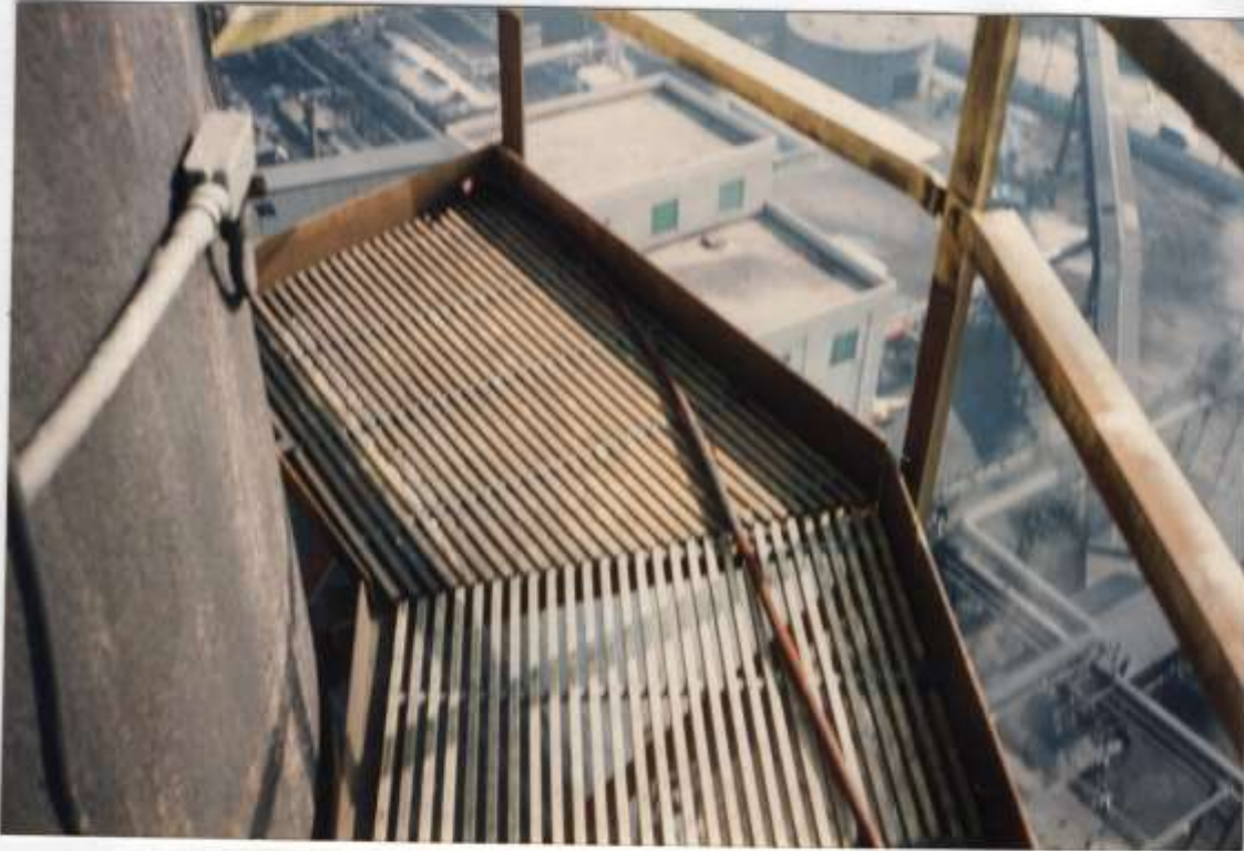
Photo # 24 View of the top platform. Minor rusting was noted.
