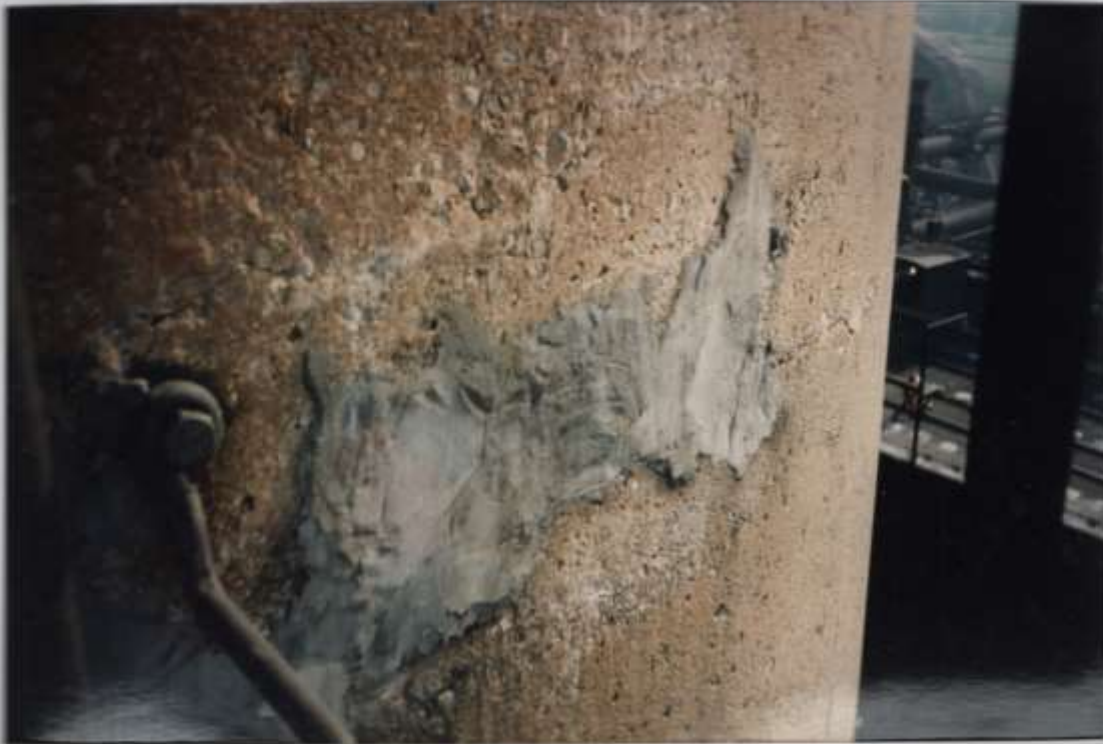
Photo #6 - Cement patch at 75' above grade elevation, right of step irons.
