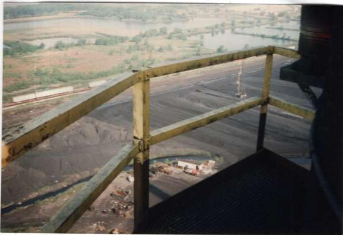
Photo #28 - Minor rusting of handrails on the top platform was noted.
