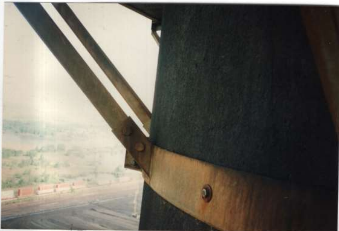
Photo #17 - The support band and bottom support angles for the top platform are all solid & sound. Minor rusting noted.
