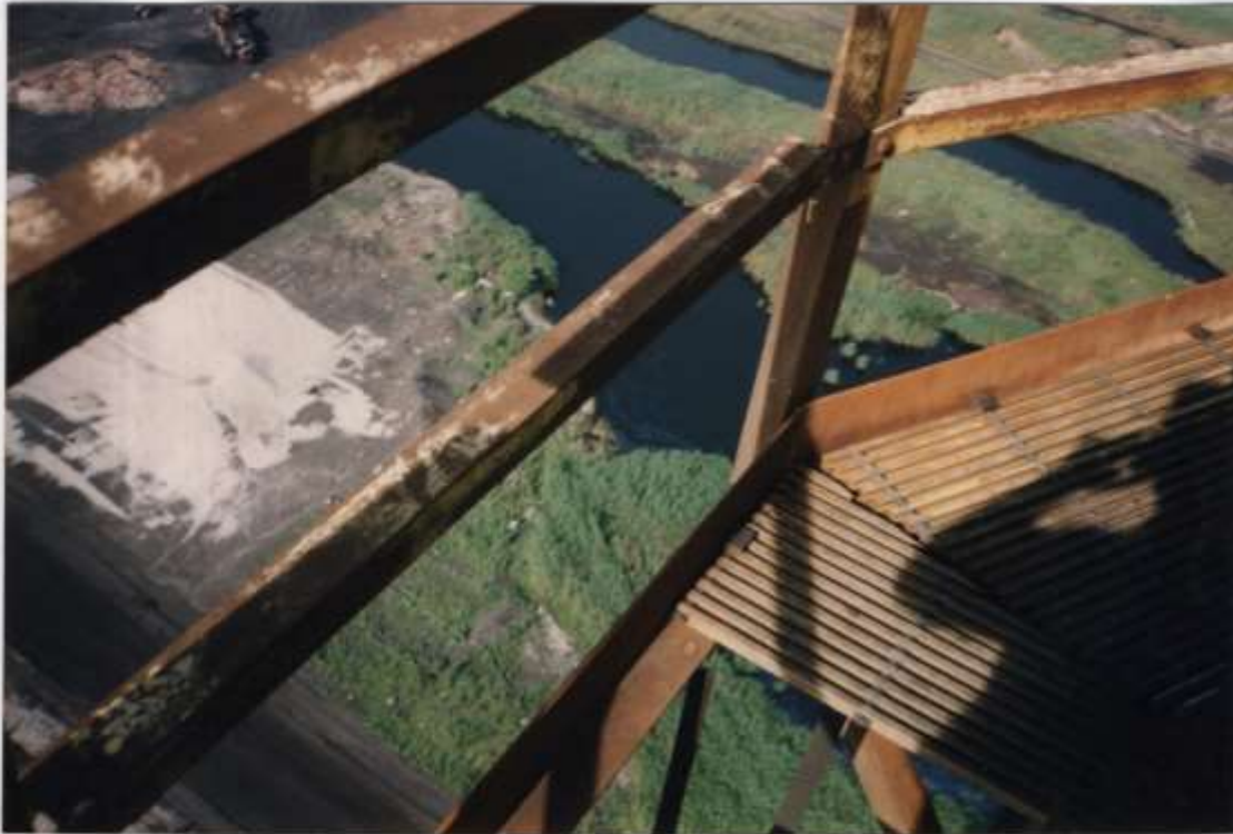
Photo #26 - Close up view of the top platform handrail. Note the steel is rusting freely.
