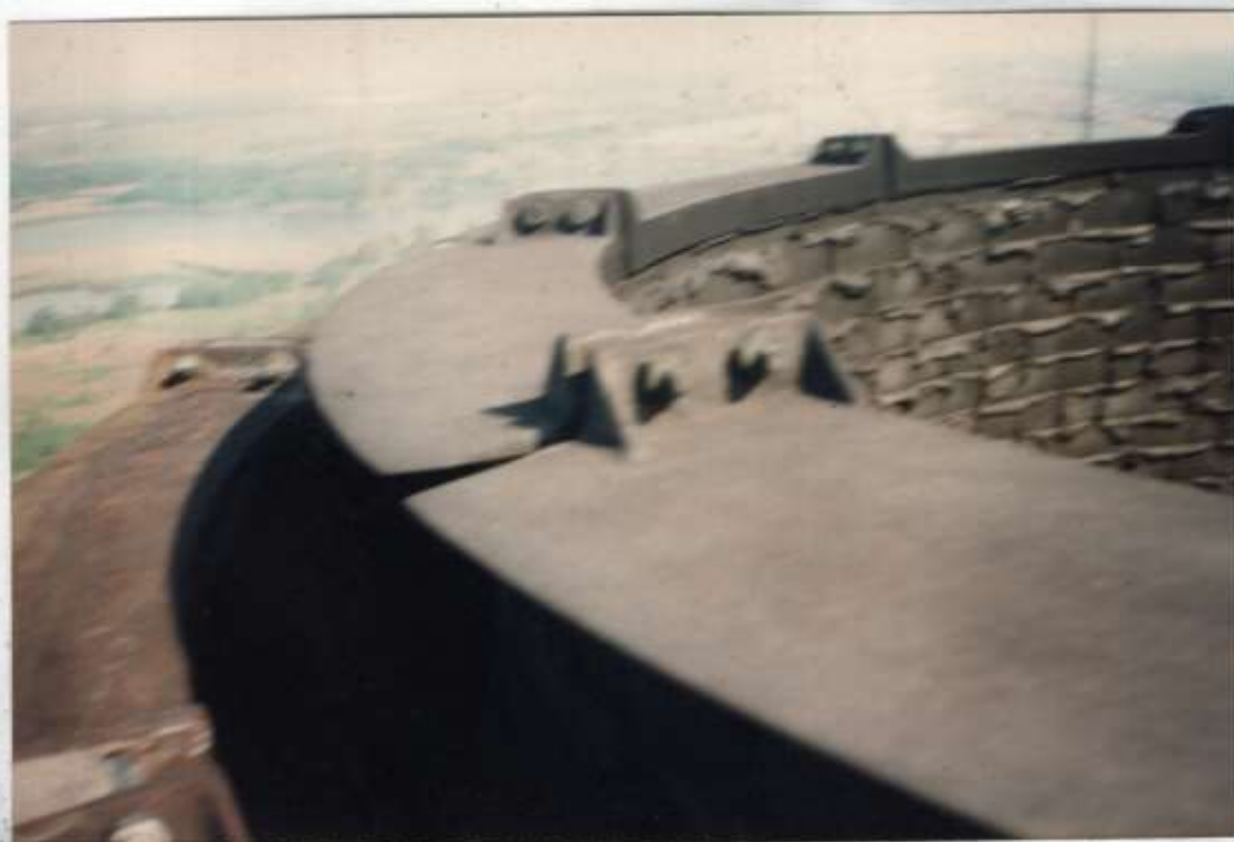
Photo #33 - Column & liner caps are intact. Note minor corrosion & rusting conditions.
