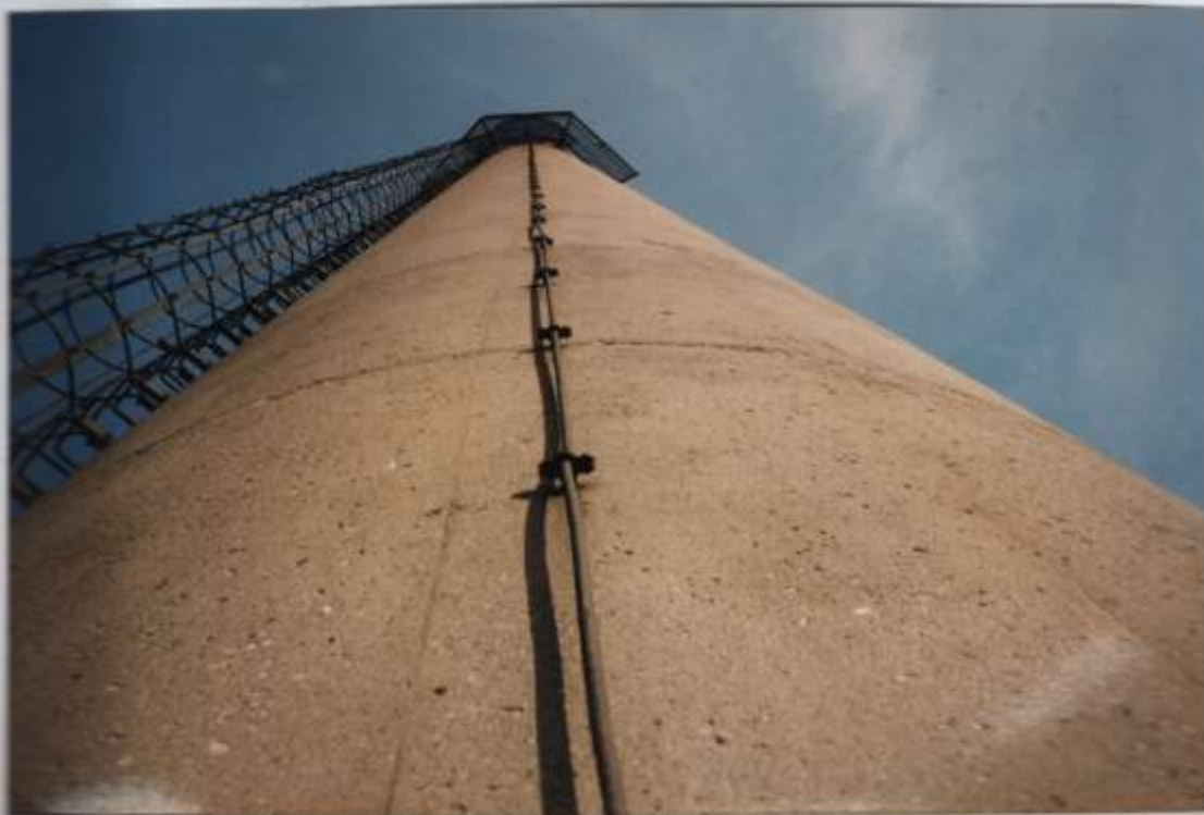
Photo #4 - View of the Lightning Protection system download cable on the east quadrant from grade elevation.
