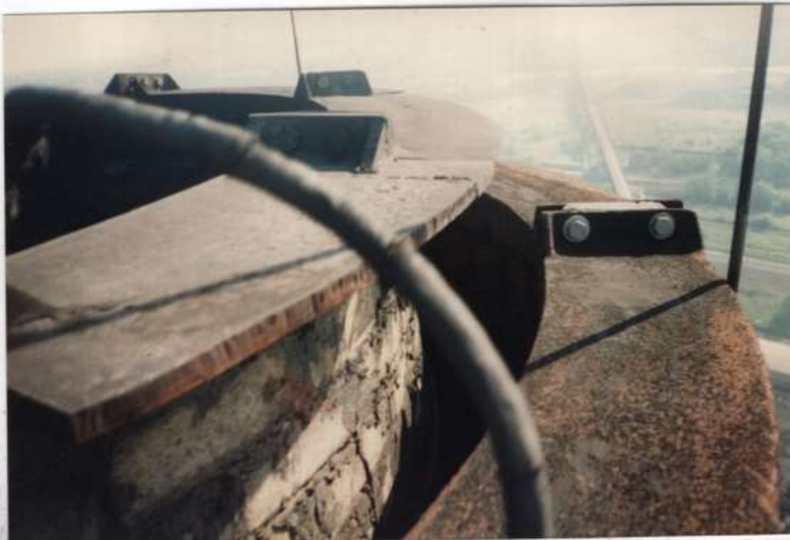
Photo #35 - Column & liner caps are intact. Note minor corrosion & rusting conditions.
