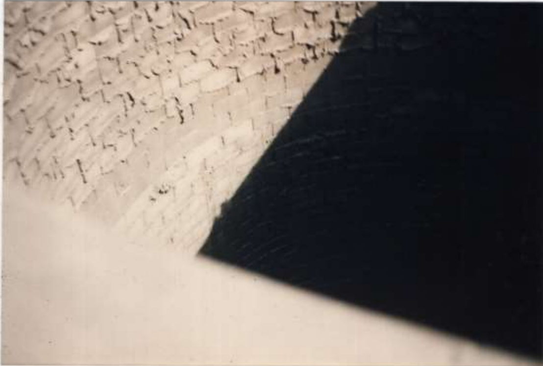
Photo #40 - View looking into the top of the liner. All brickwork is solid & sound.
