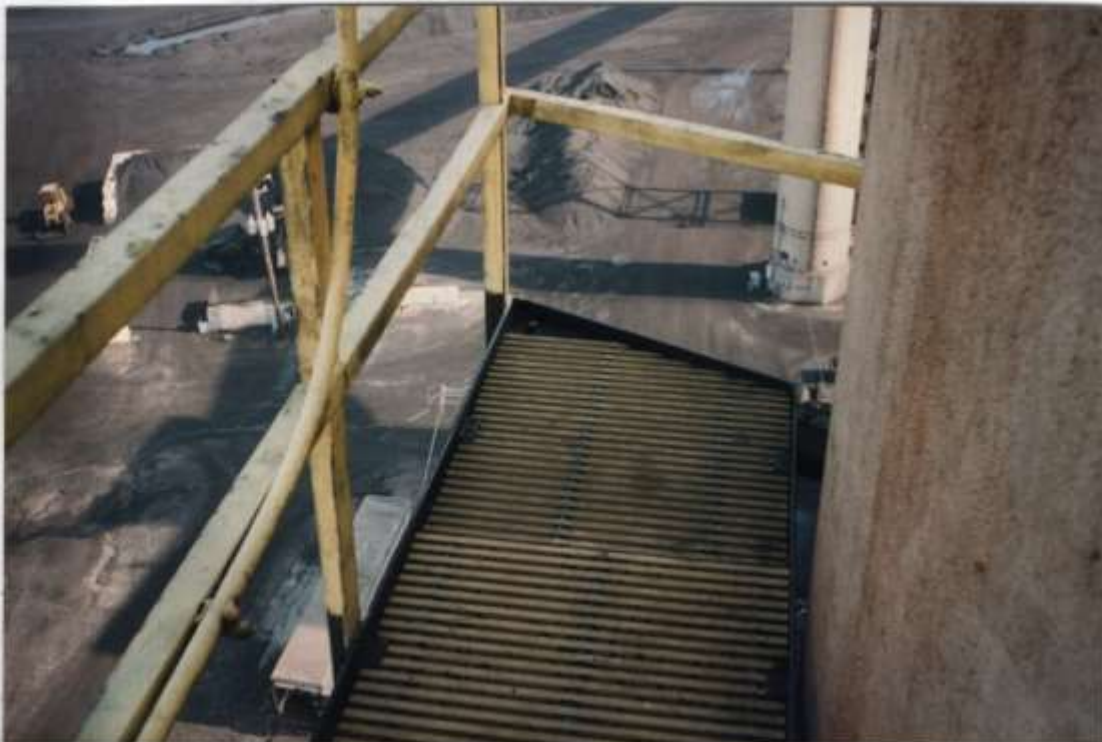
Photo #13 - Typical condition of platform at midpoint of chimney, west quadrant. Minor rusting of hand rails noted.
