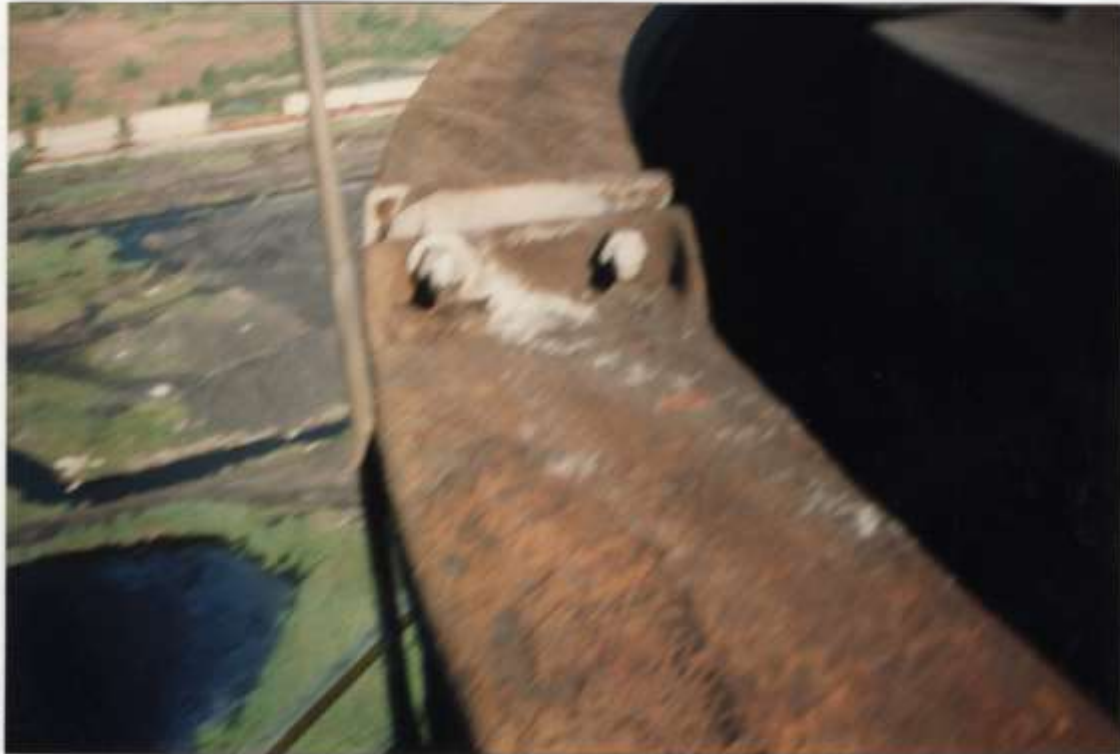
Photo #36 - Column & liner caps are intact. Note minor corrosion & rusting conditions.
