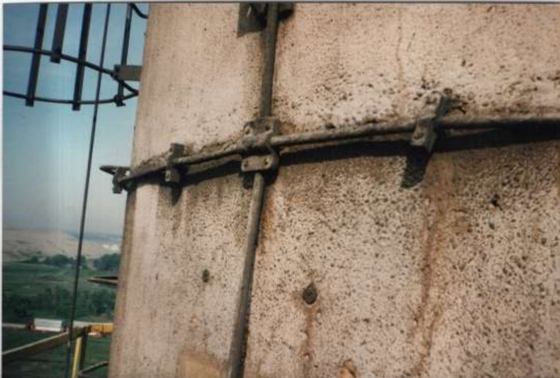
Photo #9 - Midpoint circular cable at connection to downlead, east quadrant. Note broken anchors.
