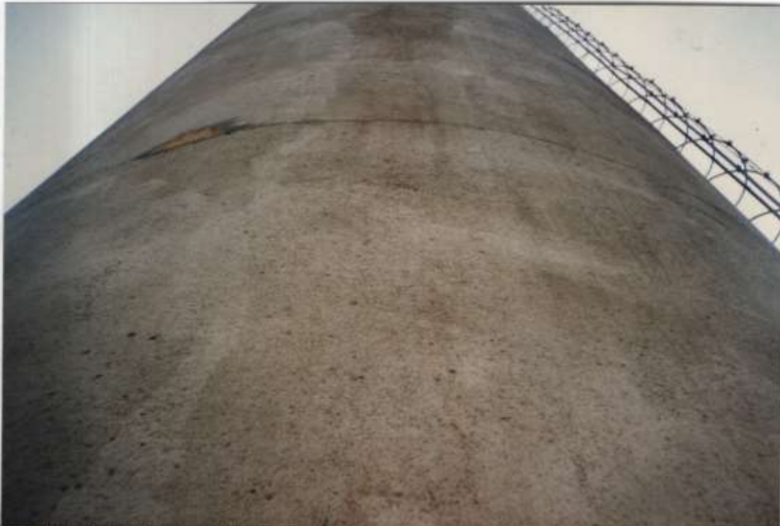
Photo #15 - Typical condition of concrete column, east quadrant. Concrete is solid & sound.
