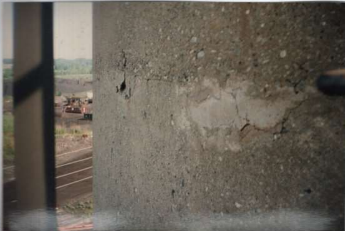
Photo #5 - View of cement patches at 50' above grade elevation. Note fractures and spalling of patch material.
