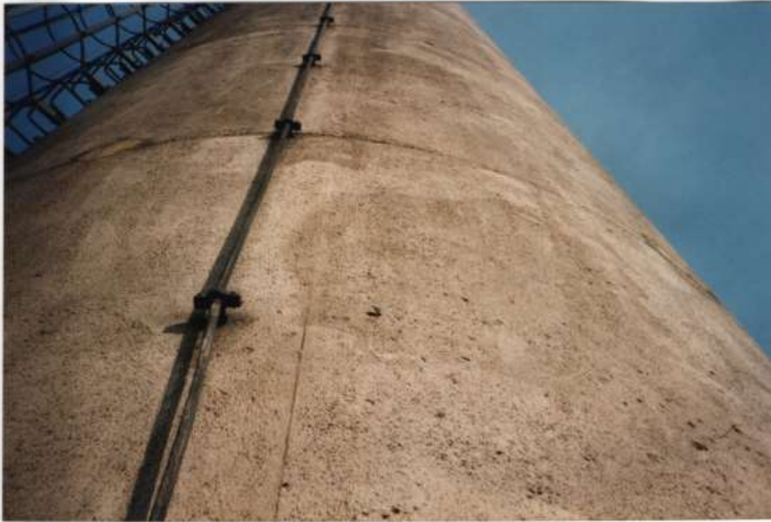
Photo #14 - View of Lightning Protection system download from mid-platform.
