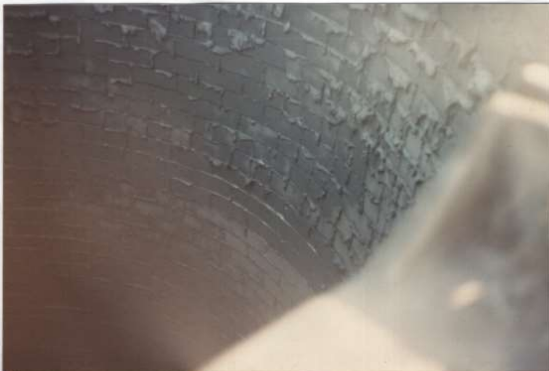
Photo #41 - View looking into the top of the liner. All brickwork is solid & sound.
