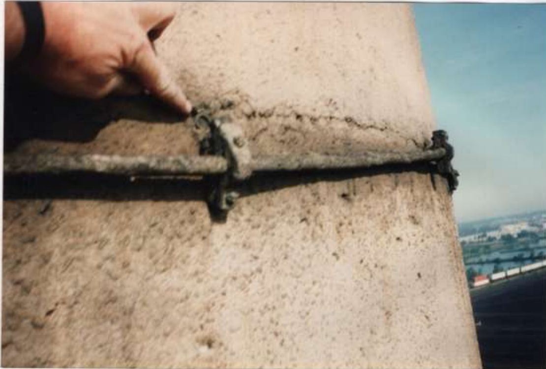
Photo #10 - Close view of the broken anchor, east quadrant, on midpoint of circular cable.
